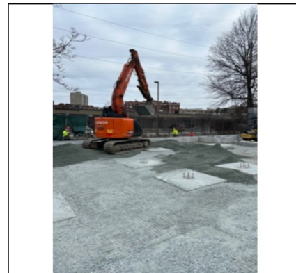
Photo FR17.5 Excavator spreading fill material at the interior of the foundation.
